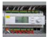
Controller box upgrade
