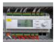
Controller box upgrade
